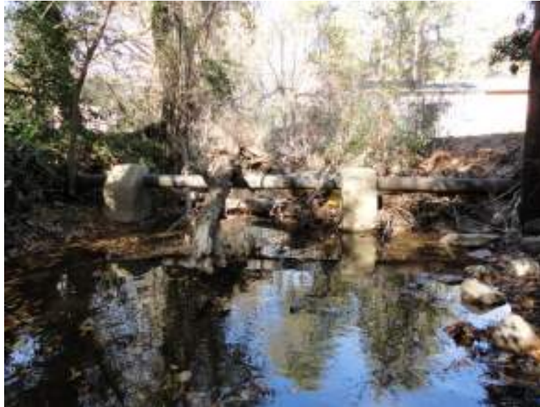
Pipe crossing Kinley Creek with collected debris, immediately upstream of K-2 confluence.
